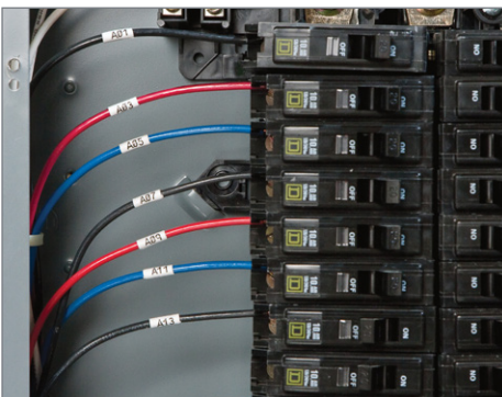
Wire and Cable Labels
